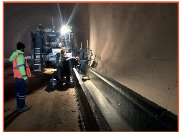
Cable Duct Application
